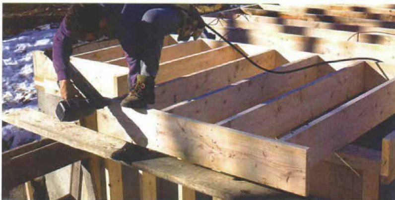
Outer rim joist is left long. Rim-joist stock is nailed to the cantilevered joists and left long until cutlines are transferred from the plates.
